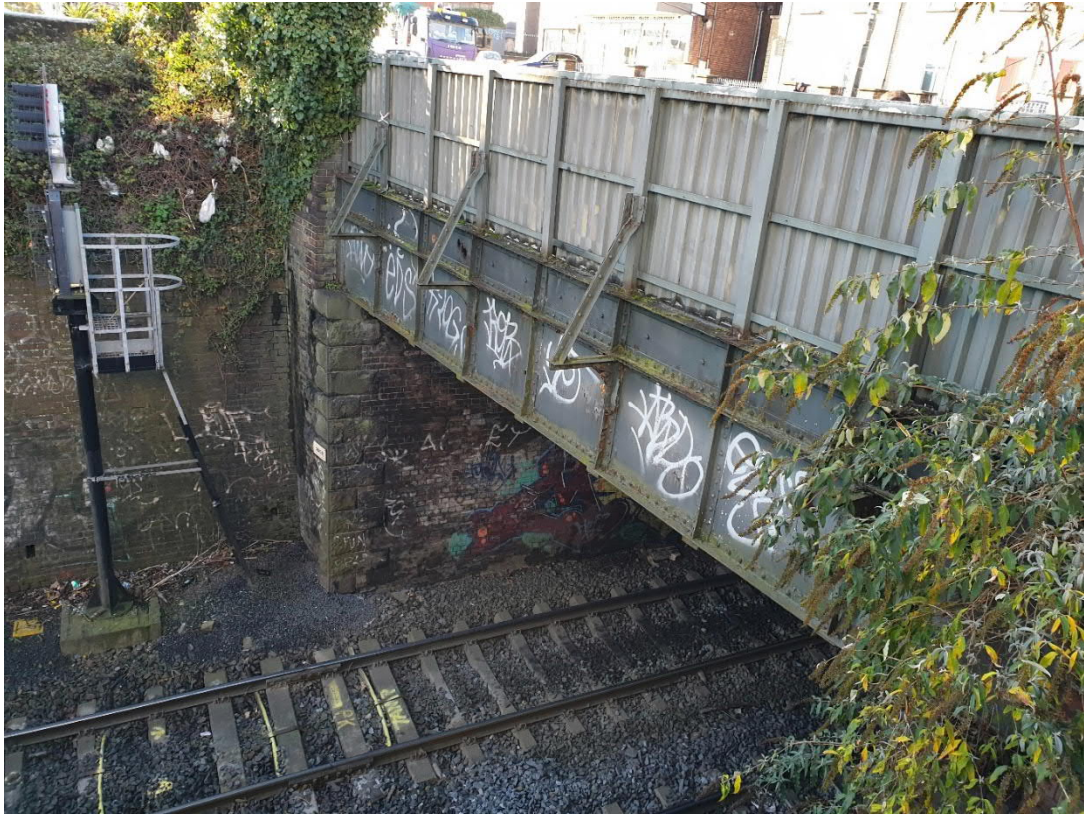
Existing Bridge (OBO11) and Parapet to be removed for bridge widening – Looking from North side
