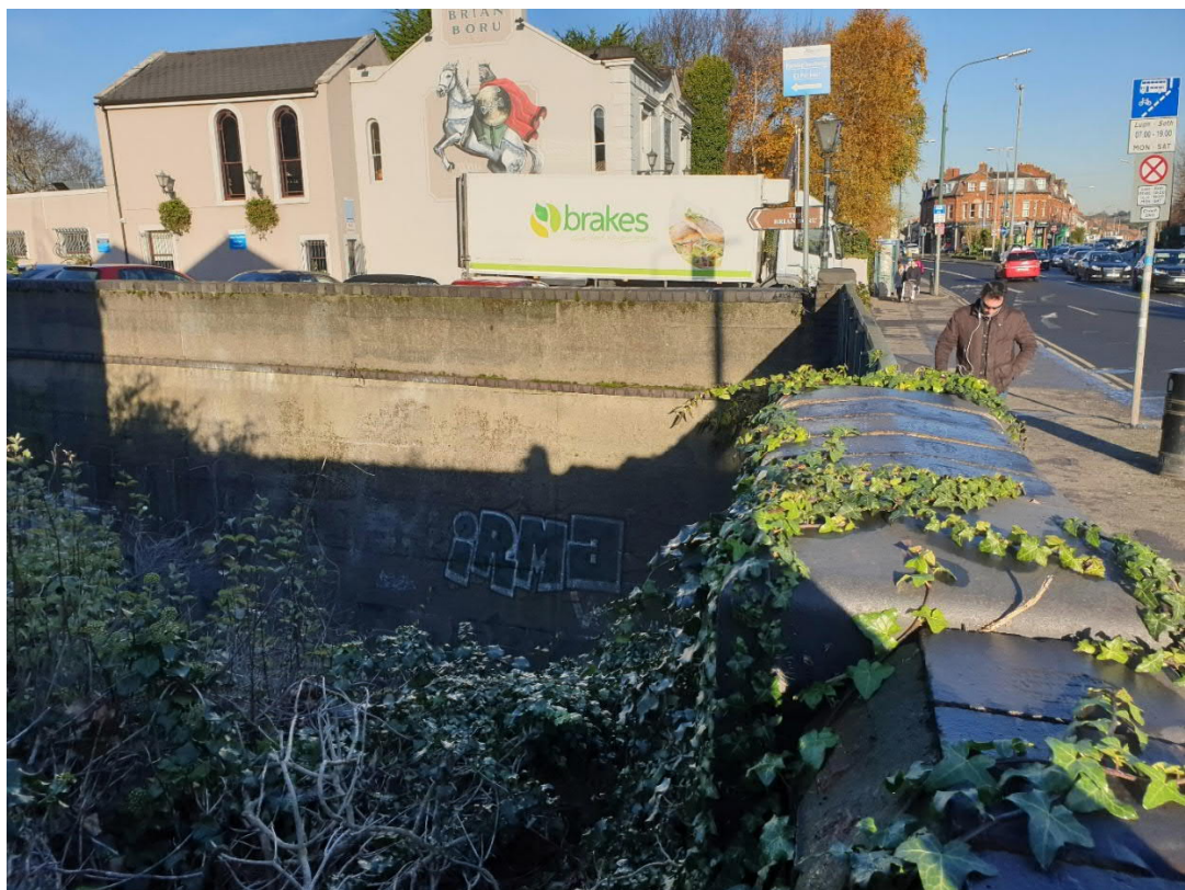
Existing retaining wall to be partially demolished due to the new bridge
