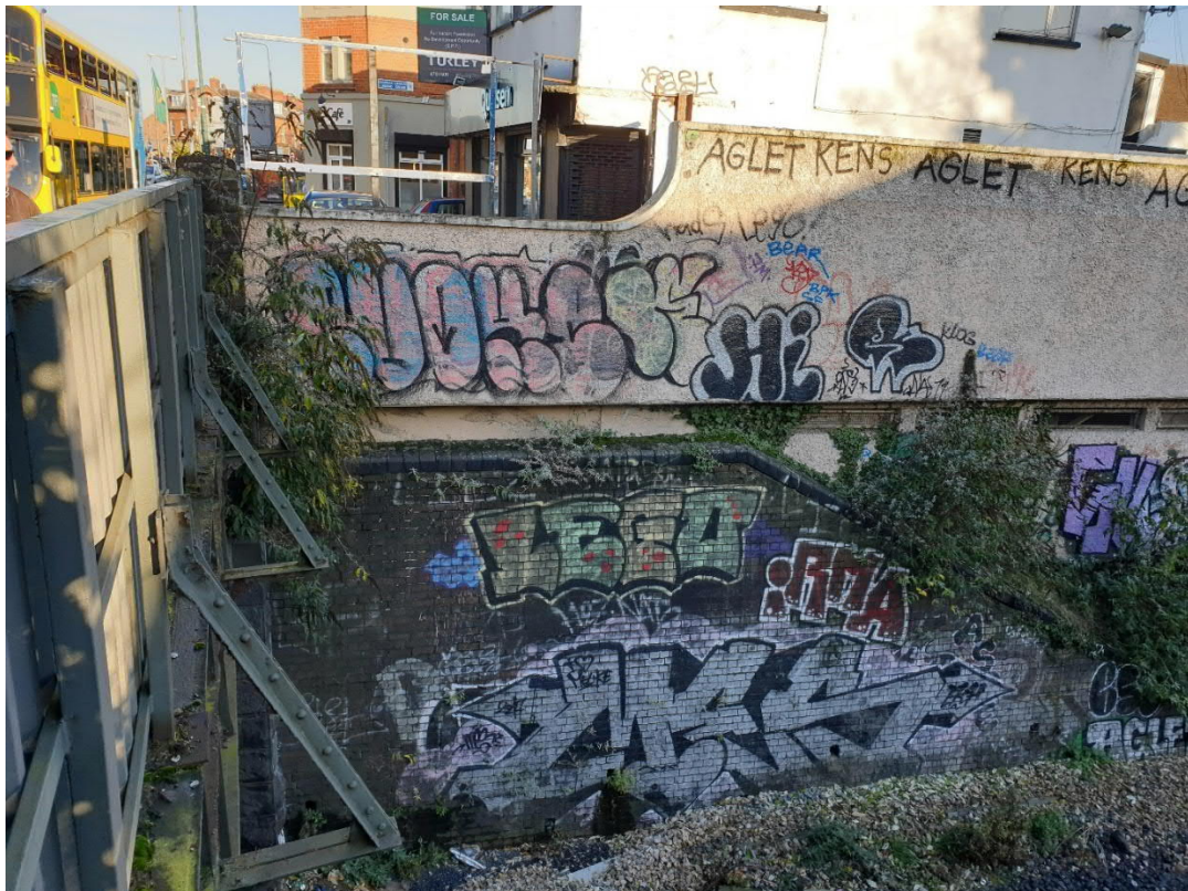
Existing Bridge (OBO11) and Parapet to be removed for bridge widening – Looking from South side
